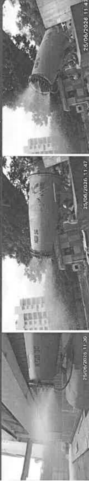
A. SMOG GUNS IN OPERATION (CONTINUOUS DUST SUPPRESSION)
